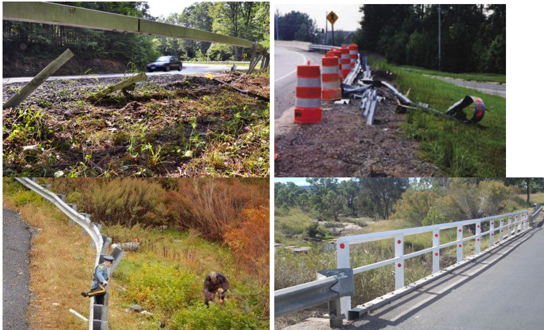
Figure 2. Examples of damaged guard rails, clockwise from upper left: (a) at the site of a fatal motorcycle accident in New York (2012), (b) damaged rails from a single-car crash (2011), (c) breakaway post-rail system repair in Australia, reported to be installed for under $9000 (2012), and (d) damage from single-car impact in New Jersey (2011).
