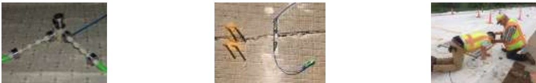
Fig. 1 Three-dimensional FRP packaged fiber optic sensors and its field installation at MnROAD, MnDOT
